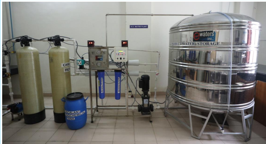
Reverse Osmosis Plant (Capacity:)
